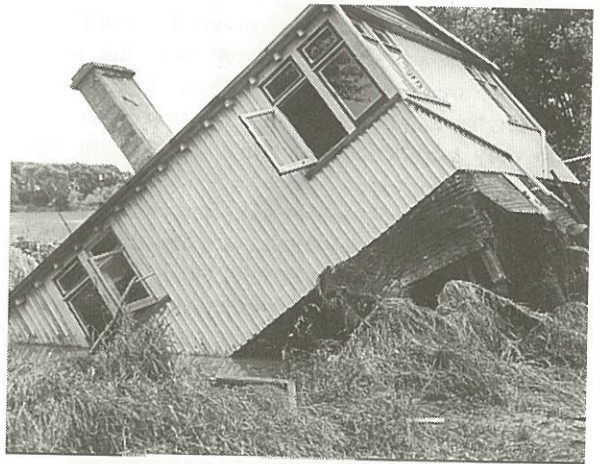
Fig. 10.6. A collapsed dwelling at Kainga, near Christchurch, after the Waimakariri River flood of December 1957. (Photo John Drew, Christchurch.)
