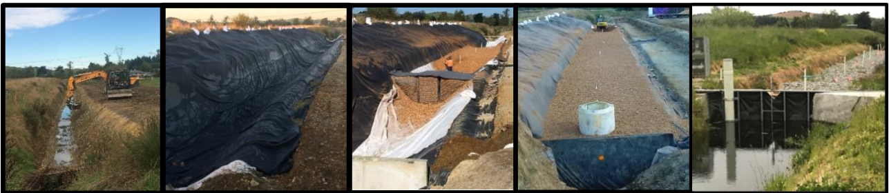
Figure 1: Photos showing various stages of the in-stream bioreactor construction. (left-right): drain clearance; laying of the EPDM rubber liner in which the bioreactor is sealed; filling the bioreactor with woodchip – concrete panel that acts as a dam end can be seen in foreground; bioreactor filled with 430 m 3 woodchip - ready to be sealed and plumbed (orange dot marks where inlet pipe was later fitted); completed bioreactor headworks – dammed drain water flows through the woodchip bioreactor under an ambient hydraulic gradient. Under storm flow conditions excess water spills over the top of the bioreactor. The white riser pipes protruding from the top of the bioreactor are monitoring wells that permit water sampling along the length of the bioreactor.
